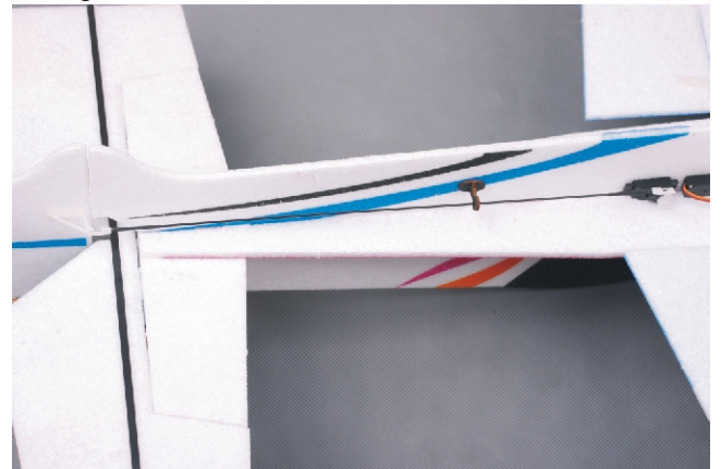
Install one control horn onto the right side of the rudder, 1" (25mm) above the bottom of the rudder. Important: Angle the control horn up toward the rudder servo, so that the pushrod will line up better.
